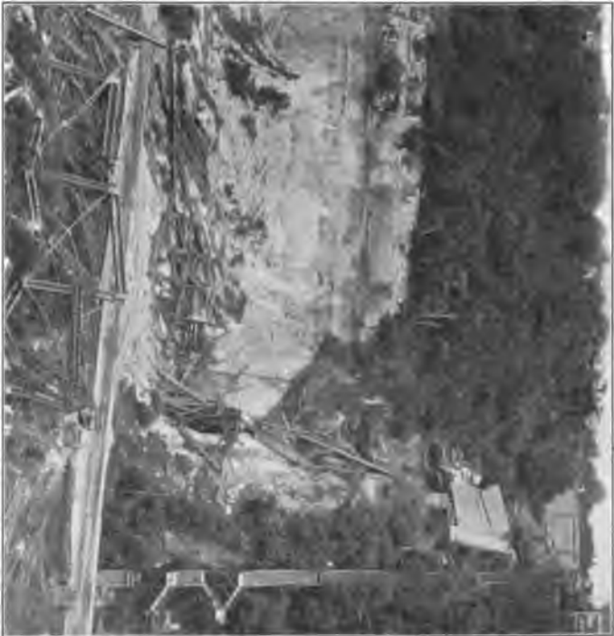
FIG. 2.—SMITH AVE. VIADUCT. VIEW FROM END OF VIADUCT STILL STANDING, SHOWING PART OF WRECK AND ABUTMENT OF WRECKED END.
